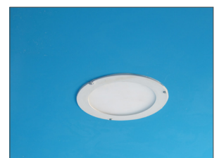
Internal recessed lights
