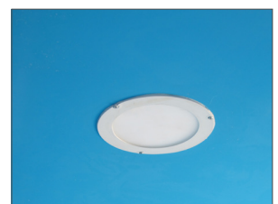
Internal recessed lights
