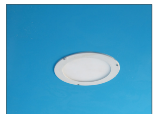
Internal recessed lights
